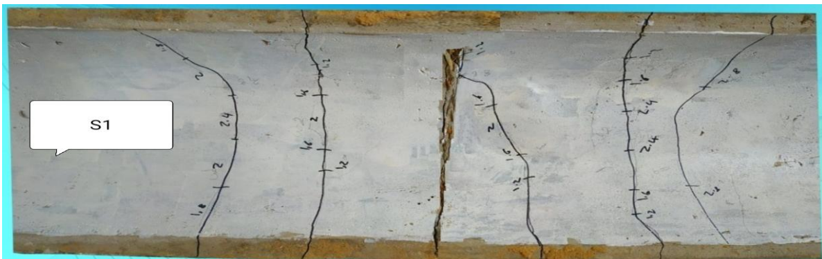
Fig. 17. Shows cracking shape of S1
