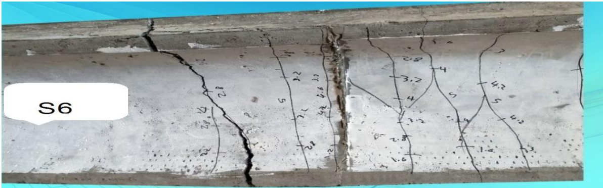
Fig. 22. Shows cracking shape of S6
