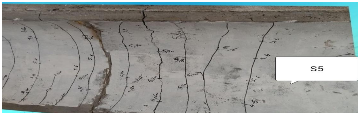
Fig. 21. Shows cracking shape of S5
