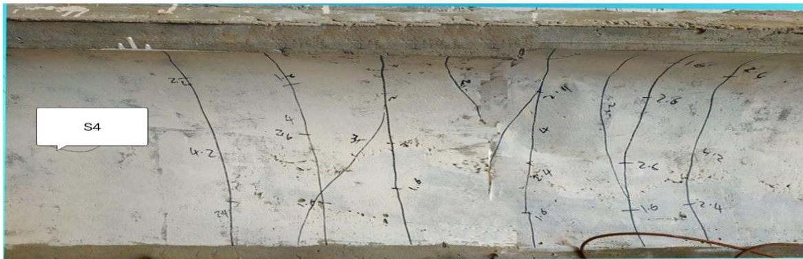
Fig. 20. Shows cracking shape of S4
