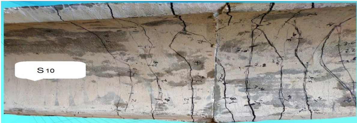
Fig. 26. Shows cracking shape of S10
