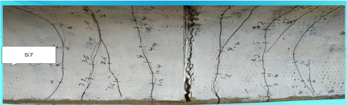
Fig. 23. Shows cracking shape of S7
