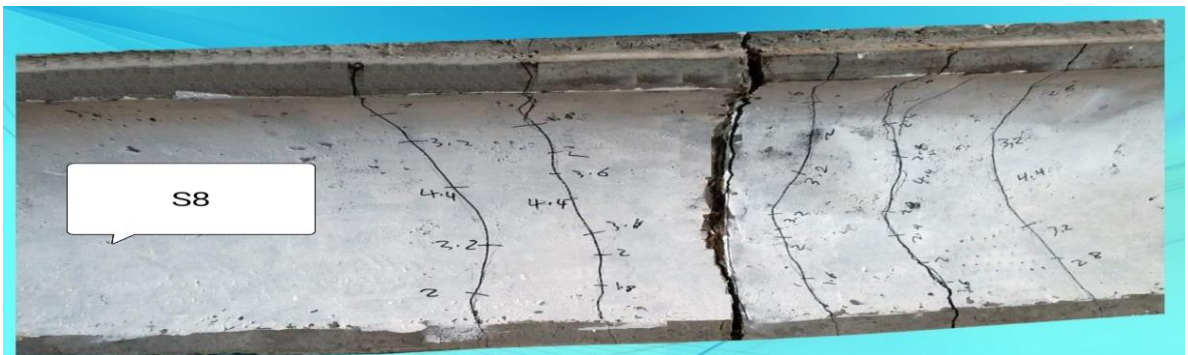
Fig. 24. Shows cracking shape of S8
