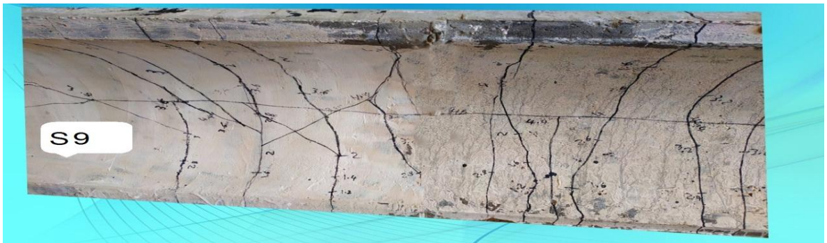
Fig. 25. Shows cracking shape of S9
